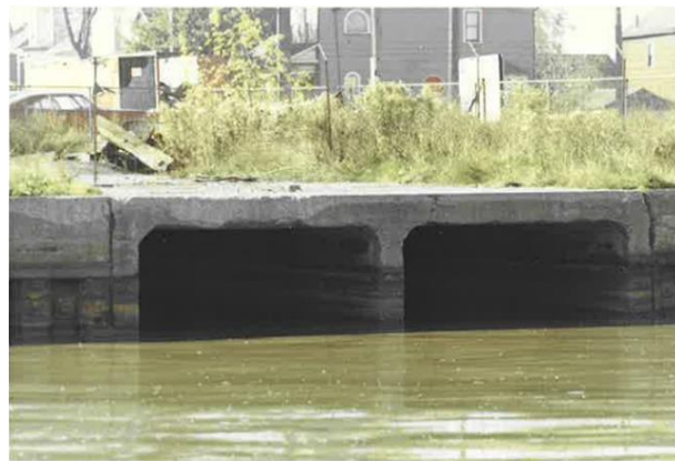
Wellington Street Storm Outfall, extremely large amounts of domestic and industrial pollution from this source, severe contamination from human excrement visible.
