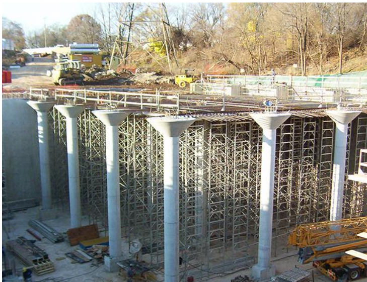
Figure 14. The City of Hamilton’s Royal Avenue combined sewer overflow tank under construction in 2007, one of several such facilities that have dramatically reduced the amount of untreated waste reaching Hamilton Harbour (Photo: City of Hamilton).
